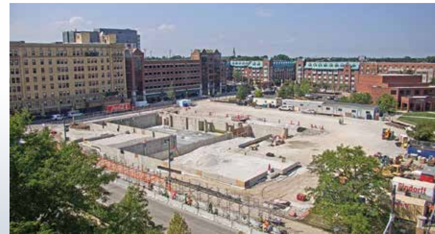
Construction is underway, and the building is scheduled for completion by the end of 2022.
